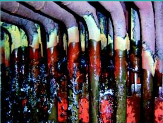
Boiler tube failure
